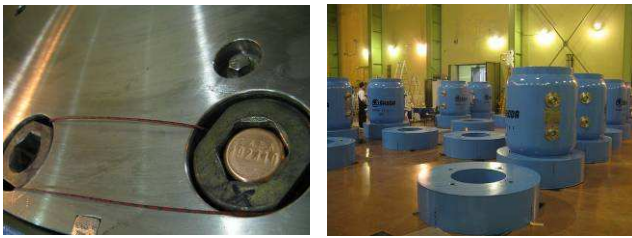
Figure 6 IAEA seal on the SKODA VPVR/M container and loaded casks in the RA reactor hall
